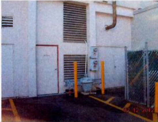
Photo #25: Exterior mounted meters on rear of the building
