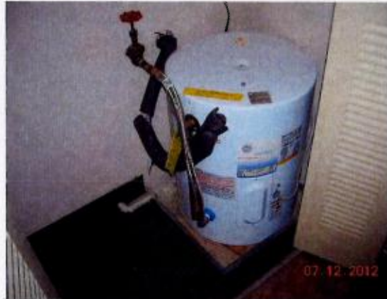
Photo #26: Closet mounted apartment electric water heater
